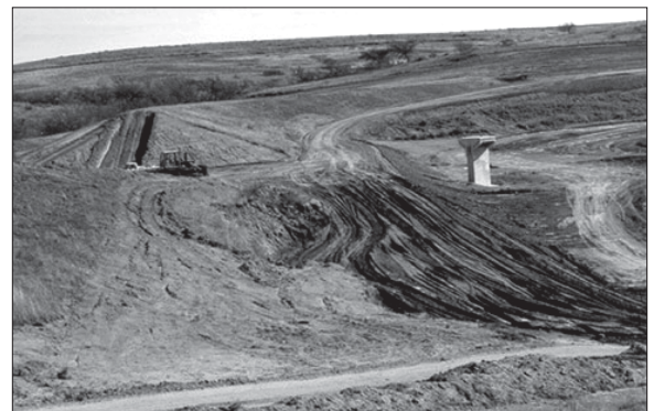
Reconstruction in April 2000 of a small flood control dam in Roger Mills county, one of 6 dams built in the Sergeant Major Creek Watershed from 1948 to 1963. This site was selected for reconstruction as a result of a hazard classification change due to downstream development, structural problems with the principal spillway, and excessive foundation seepage.
