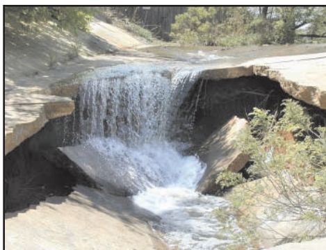
Knight Lake's crumbling spillway is indicative of numerous deficiencies in the west Oklahoma City dam.
