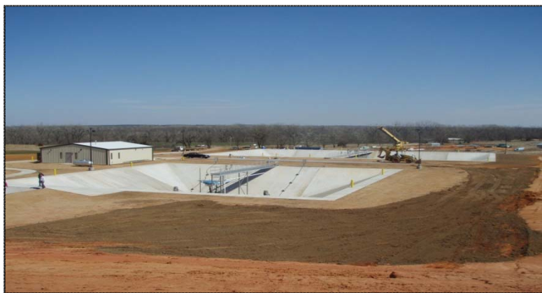
McLoud PWA New Sequencing Batch Reactor Facility financed by a $5,135,000 CWSRF Loan, McLoud, Oklahoma.
