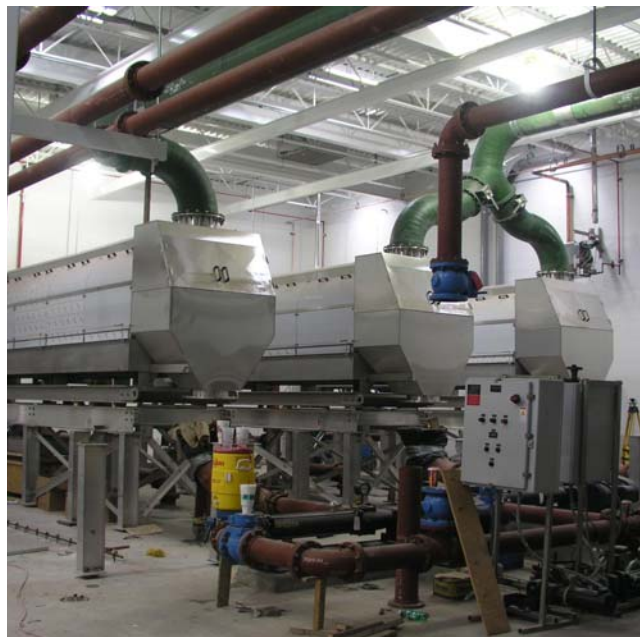
Tulsa's Southside WWTP Sludge Thickening Units
