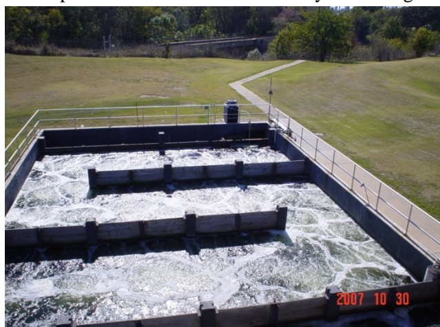
Ardmore Public Works Authority new chlorine contact basin.
