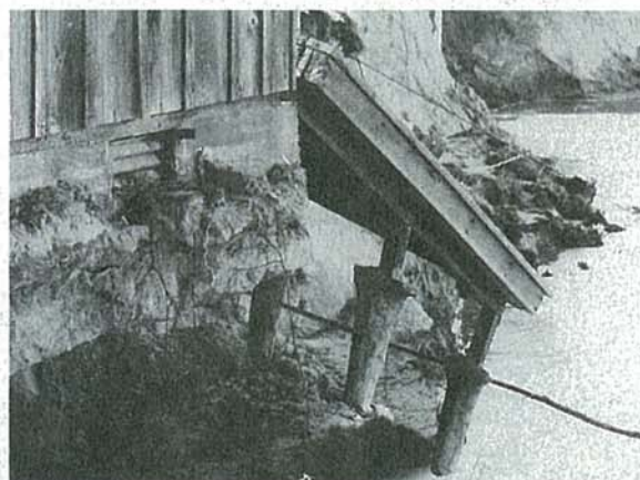
The river under cut the deck, encroached on the foundation and swept away fences, trees and septic tank.
