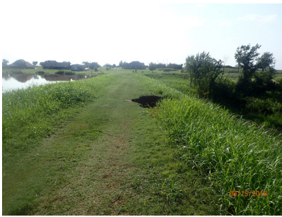
The state of the dam when OWRB Dam Safety engineers arrived on site August 15, 2018.
