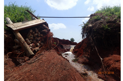
Total dam breach photographed two days after the rainfall event.
